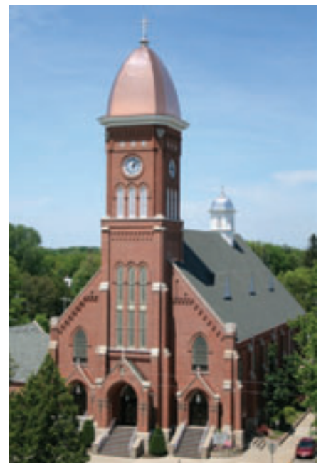
■ DECRA’s Shingle profile in Vintage Slate was installed May 2006 to help preserve the 100-year old St. Peter Catholic Church in Stevens Point, Wis. (Photo by Kulp’s of Stratford.)
